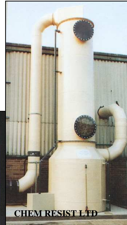
Scrubber for ventilation air
